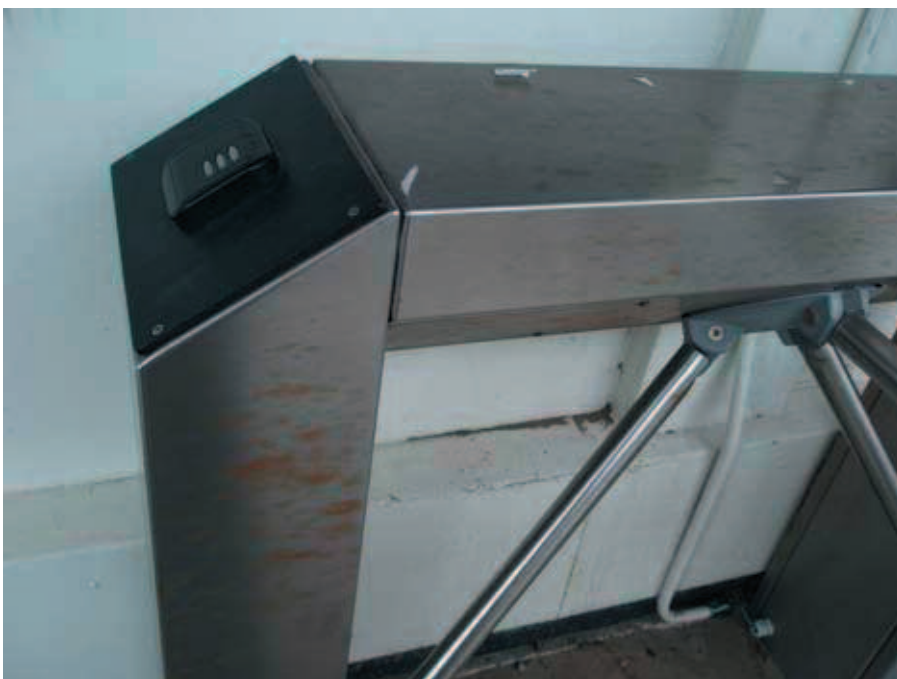
Fig. 2. RVS 316 access gate corroded by aerosols.
