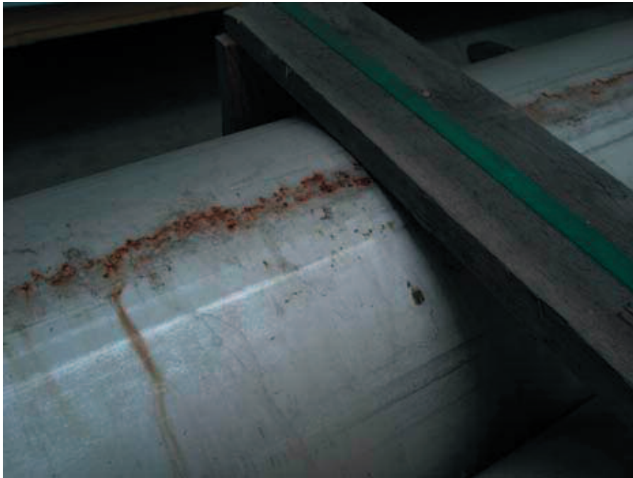
Fig. 7. Stainless steel 316 tube that was badly contaminated by steel grit on a building site.
